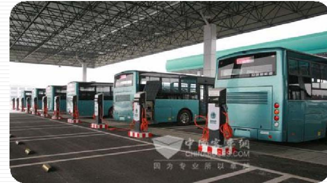
Electric charging pile
