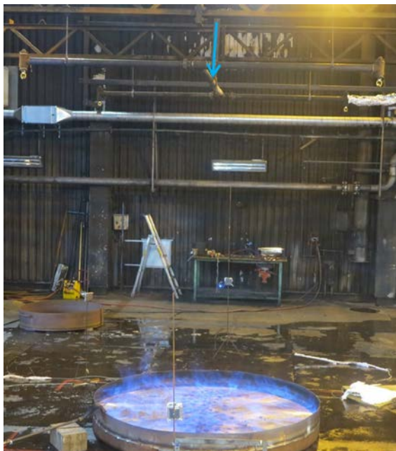
Figure 5. Hydraulically balanced water-spraying system with single feed (marked by blue arrow).
