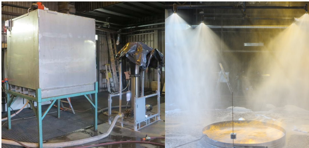
Figure 7. Water tank with premixed foam and pump (left) for the water-spraying system to provide 5 \text{ l/m}^2/\text{min} (right).
