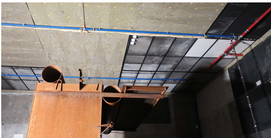
Figure 3. Pipe-work providing 3.3x3.3 m spacing between sprinkler nozzles (two branches visible).
