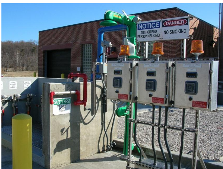
Figure 6-6. Methanol storage transfer station
