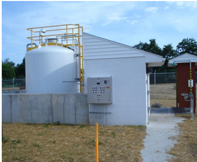
Figure 6-3. Steel tank with concrete secondary containment 7
