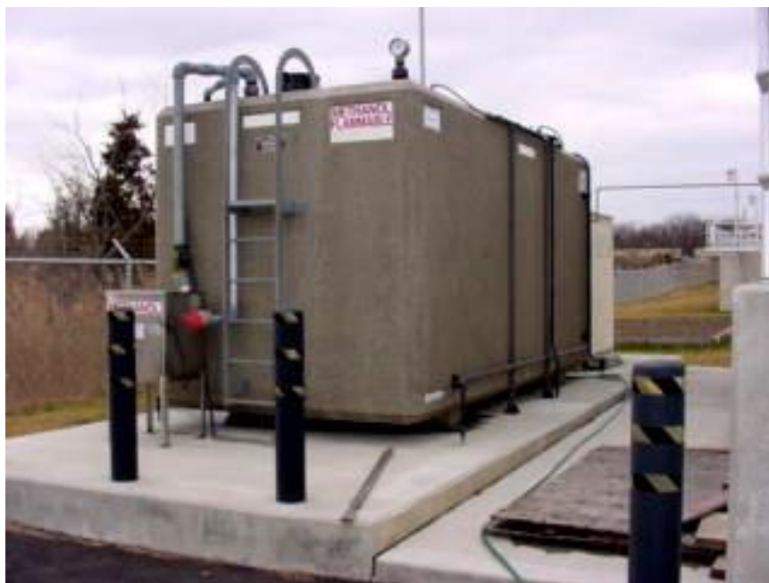
Figure 6-4. Double contained concrete tank with steel inner tank (no additional containment required) 8
