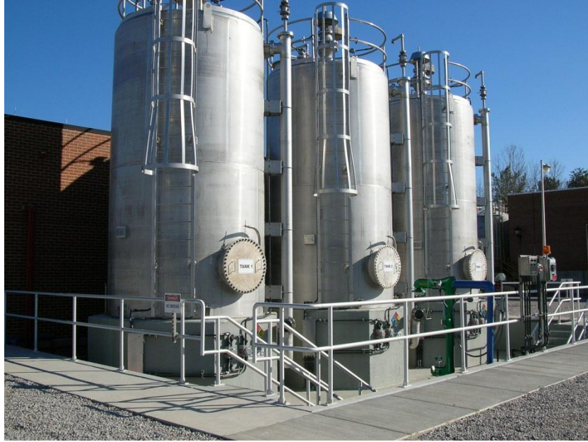
Figure 6-2. Large methanol storage tanks with secondary containment
